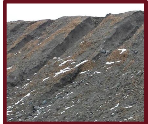
Slope with failures. Sides are too steep and are not well packed.
