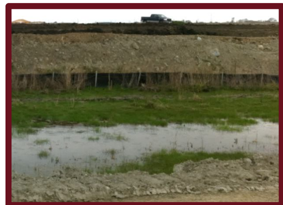
Fill applied in thin layers, with a silt fence at the base of the fill. Grass is maintained on the edge of the drainage.
